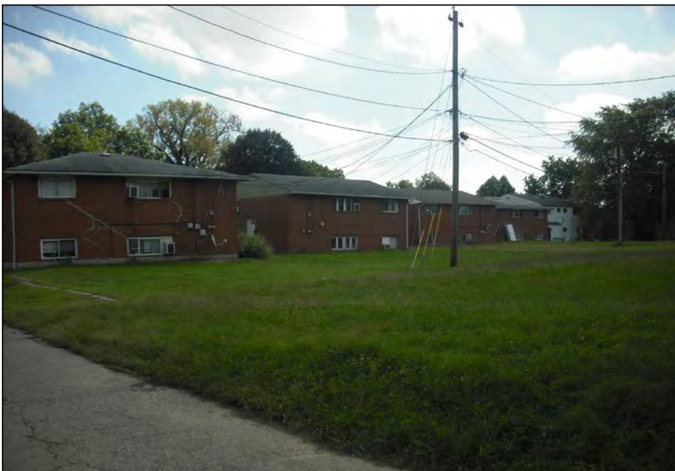
View of the multi-family residences located on the eastern portion of the subject property along Ferndale Place. Note the cracking and patches in the building foundations and uneven terrain in the shared yard space.
