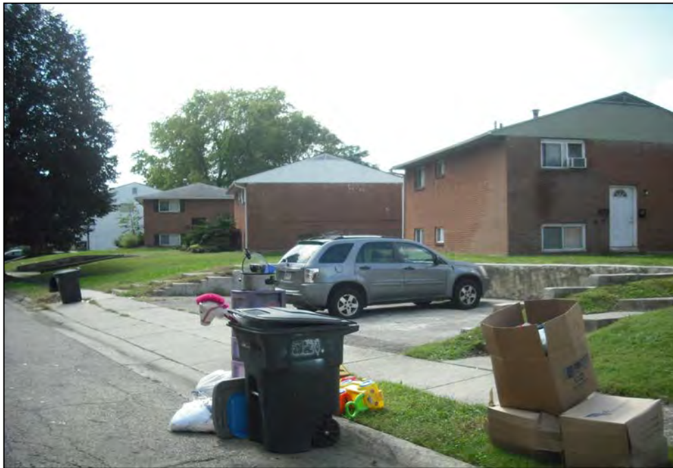
View south along Ferndale Place of the on-site multi-family buildings and parking spaces servicing the dwellings. Note the cracked concrete and uneven terrain of the walking paths leading to the on-site buildings.
