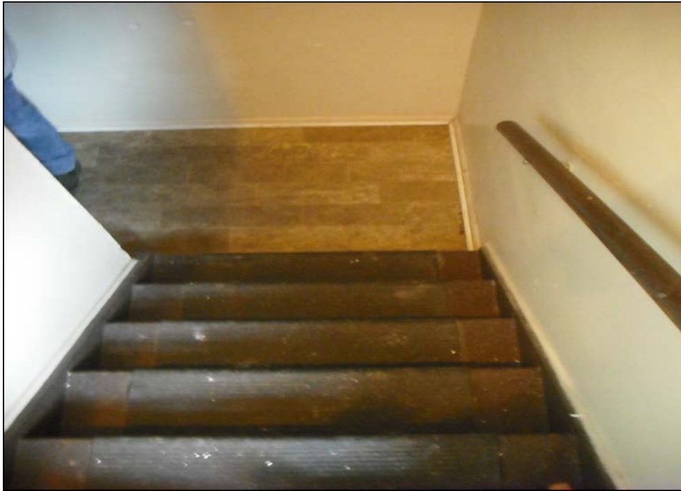
View down the staircase from the landing of the entryway into the 945 Ferndale Place building. Two units are located in the building. One in the basement, and one on the 2nd floor.
