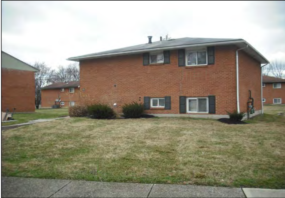
View west of 921-925 Ferndale Place. Note the uneven and dipping terrain around the building.
