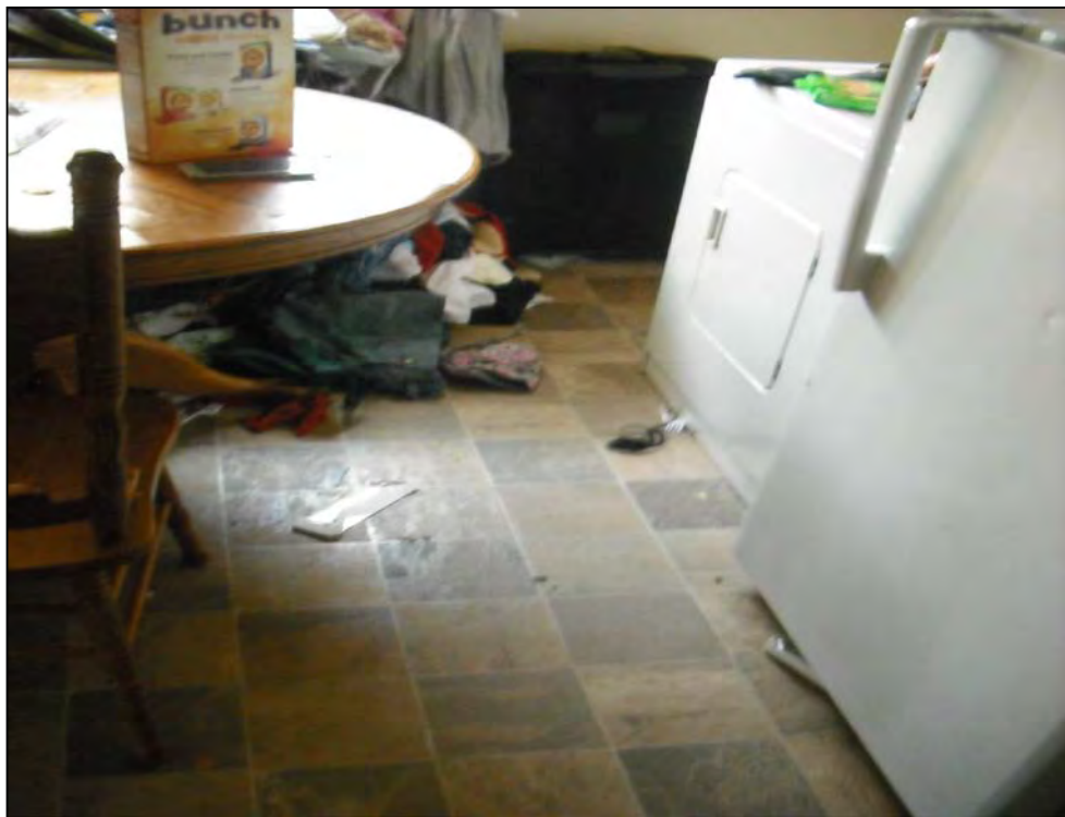
Laminate flooring in the kitchen area of the 2nd story unit (Unit B) of the 945 Ferndale Place building.
