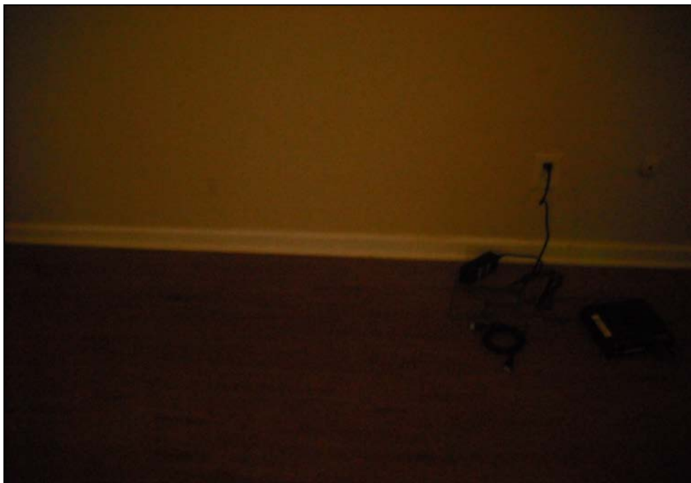
Wood panel flooring in the basement unit (Unit A) of the 945 Ferndale Place building.
