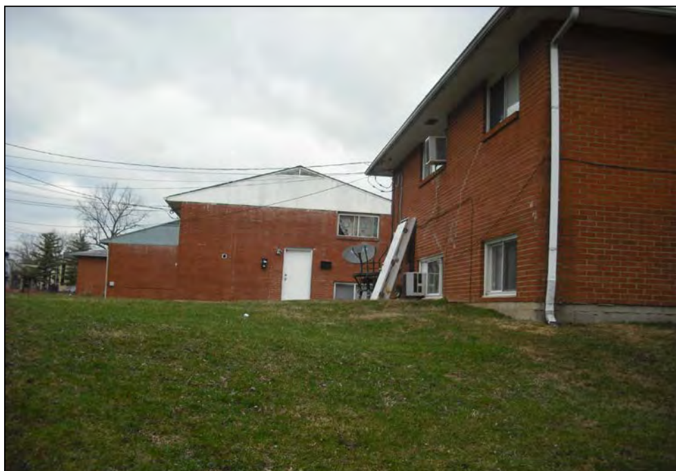
View north from the south side of 945 Ferndale Place. Note the elevation change and uneven topography of the property. Visual cracks in the building are observed which are a sign of subsurface movement / settlement.
