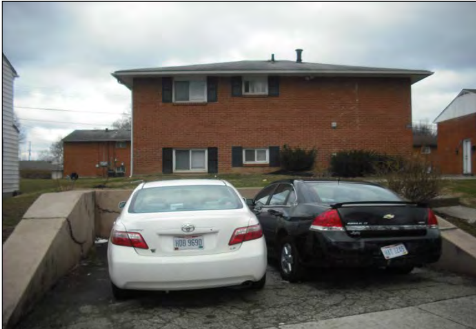
View west of the front of 941-945 Ferndale Place residence. Note the cracking and signs of settlement / subsurface movement in the parking barriers and pavement.
