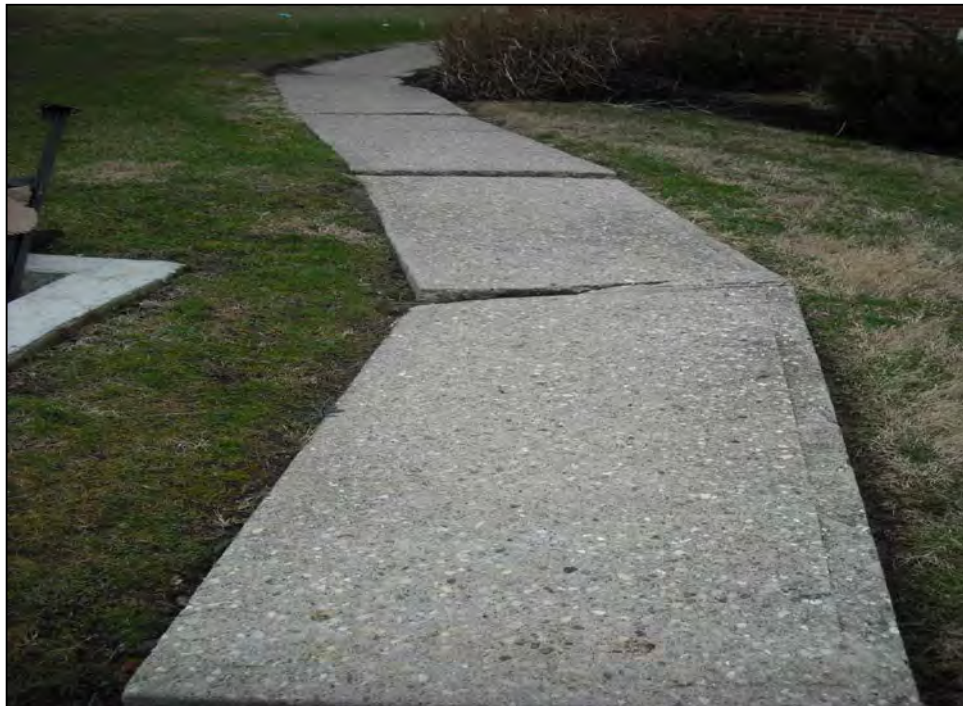
View west of the entryway to 921 Ferndale Place. The sidewalk shows signs of settlement / movement in the subsurface.
