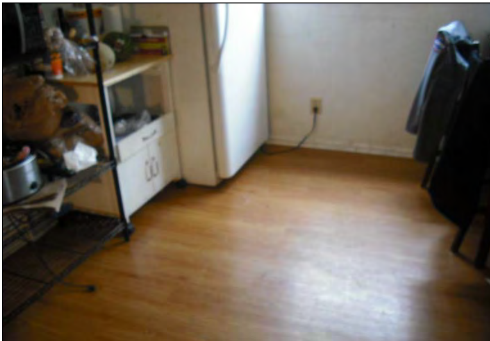
Wood panel flooring in the basement unit (Unit A) of the 921 Ferndale Place building.
