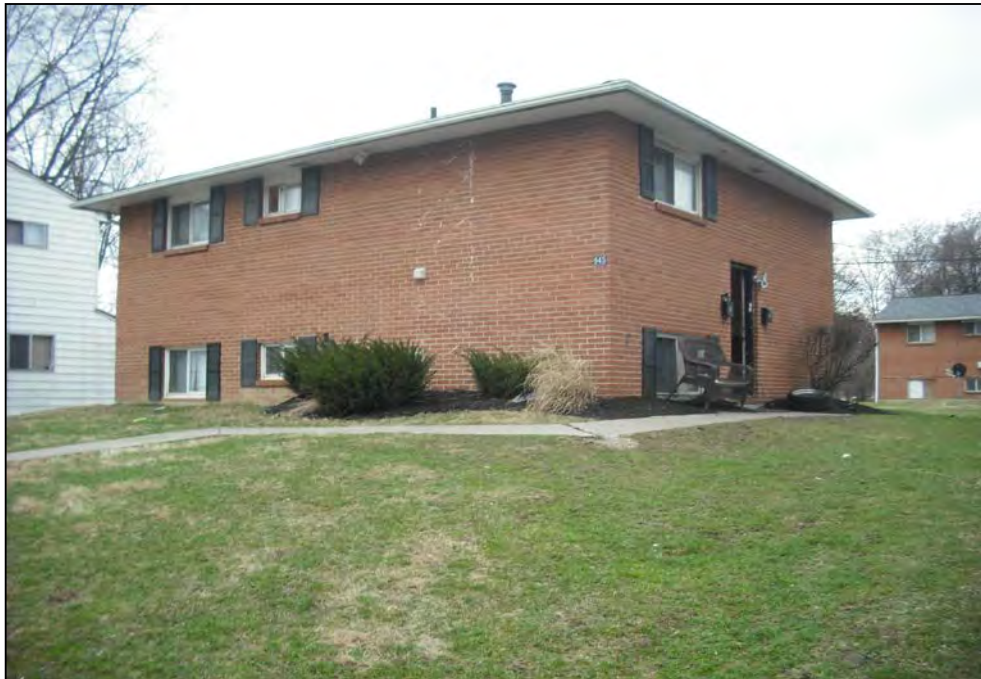
View west from Ferndale Place of the 945 Ferndale Place residence. Note the uneven, and dipping terrain surrounding the building which shows sign of settlement.
