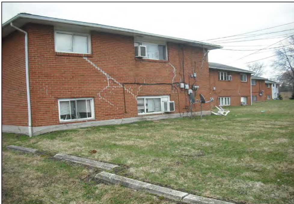
View southeast of 921-925 Ferndale Place building. Note the visual cracking in the building foundation and walls which show signs of movement / settlement.
