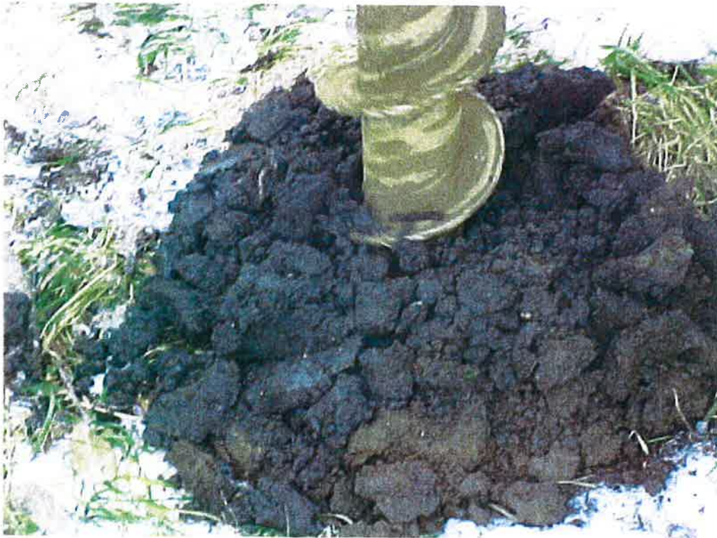
Photograph 6: View of soil clippings from geo-technical boring containing glass and metal fragments.
