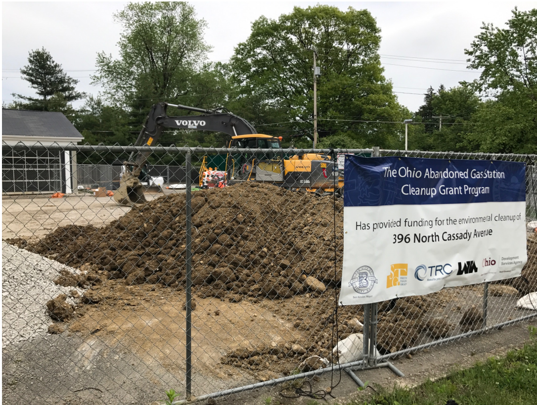
Sunoco on North Cassady Cleanup in Progress
