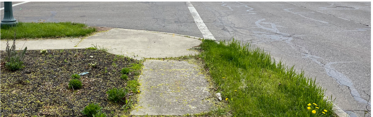
Unsafe pedestrian/sidewalk conditions
