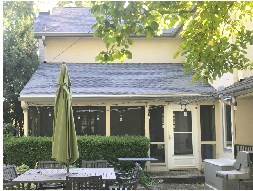
Bottom of Wall to be raised to 18". Screens to be replaced with Pella 250 sliding windows. Door to be replaced with sliding door. See Page 4
