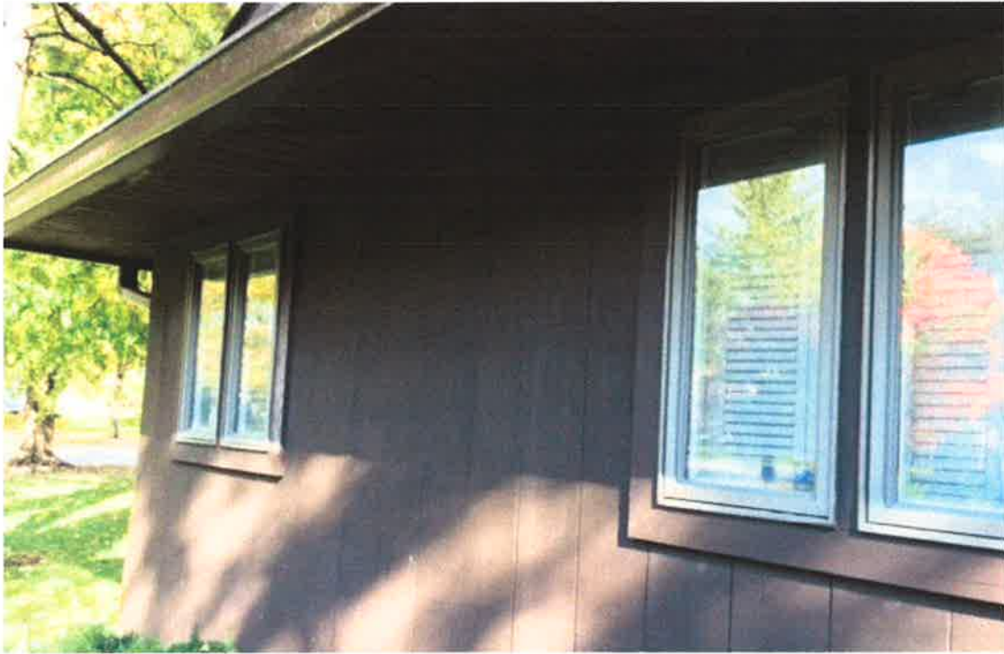
Detail of the trim work around the existing windows of the house to be incorporated into the panel detail.
