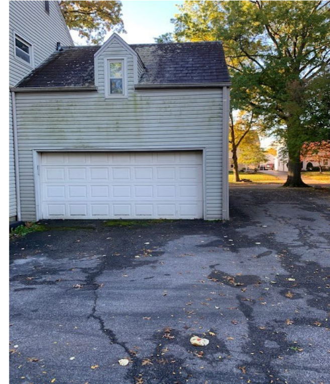
Pic #3: Garage not functional due to size
