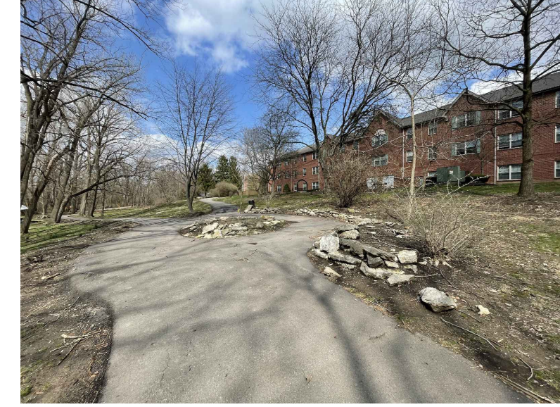
EXISTING ROUND ABOUT. ALL STONE TO BE REMOVED. VERIFY ON SITE REMOVAL OF PLANT MATERIAL.
