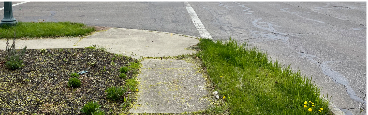
Unsafe pedestrian/sidewalk conditions
