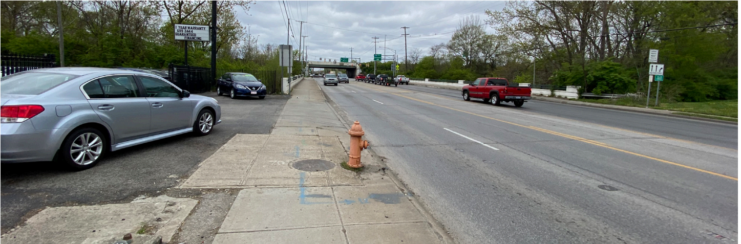
Unsafe pedestrian/sidewalk conditions
