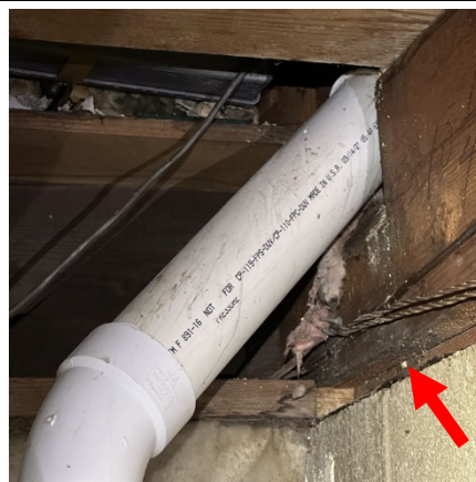
Rim board water infiltration at corner
