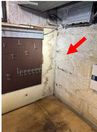
Water infiltration at CMU wall corner
