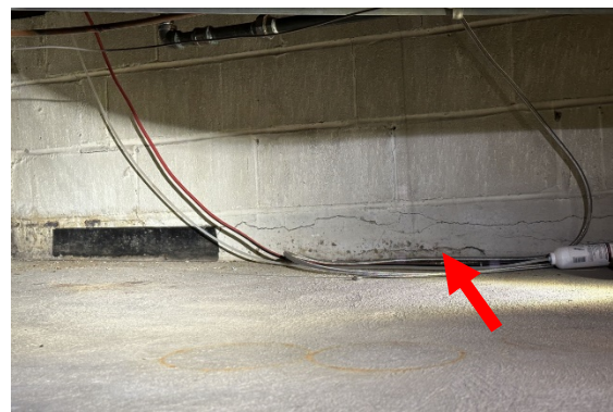
Concrete lintel cracks due to internal corrosion
