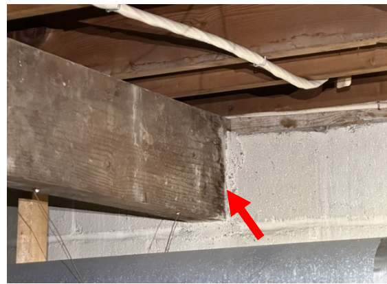
Beam water infiltration at end
