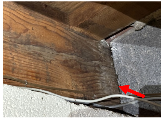
Rim board water infiltration at corner
