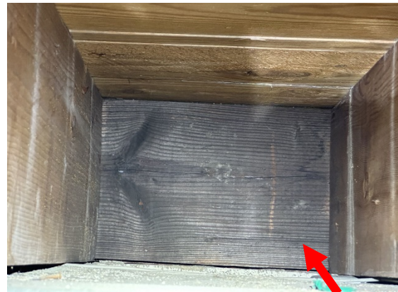
Rim board discoloration
