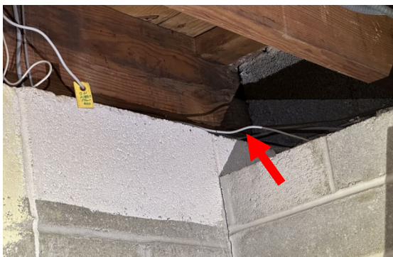
Rim board water infiltration
