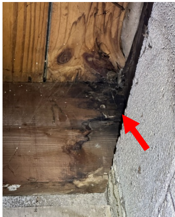
Rim board water infiltration at corner
