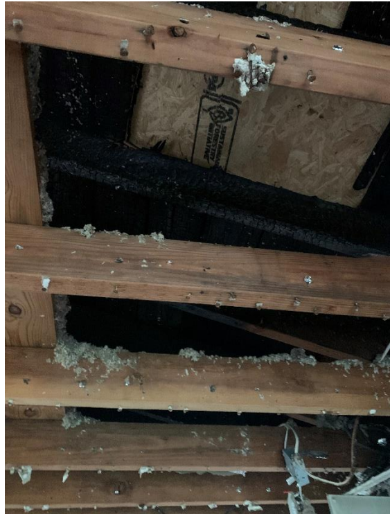
Figure 2. Kitchen Fire Damaged Roof Trusses
