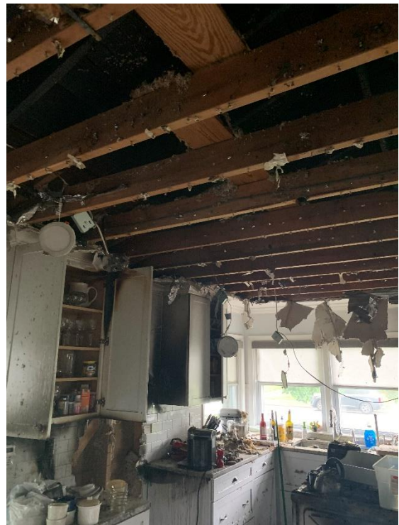
Figure 4. Kitchen Fire Damaged Roof Trusses
