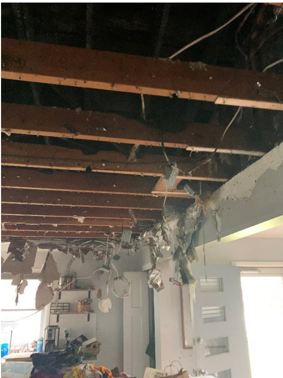
Figure 3. Kitchen Fire Damaged Roof Trusses
