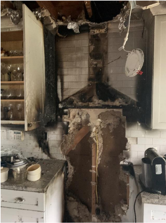
Figure 1. Kitchen Stove Area Fire Damage
