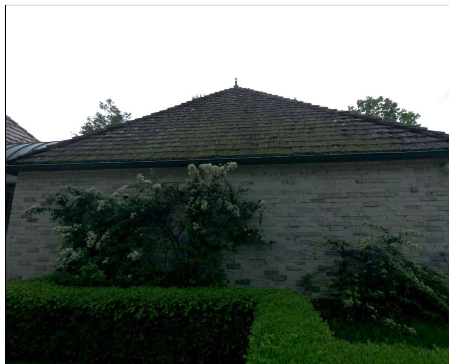
B GUEST SUITE - NORTH EXTERIOR ELEVATION - LOOKING TOWARD PROPOSED WINDOWS SCALE: NTS
