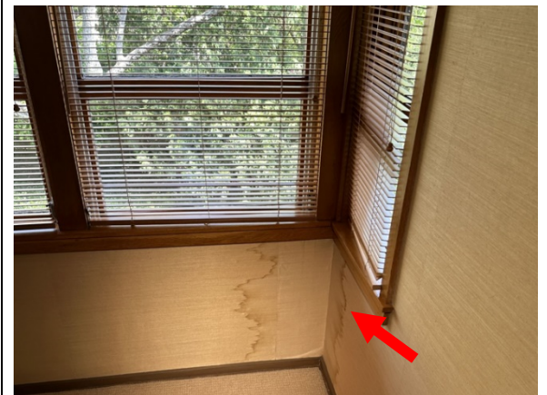
Water infiltration at north side wall / low roof
