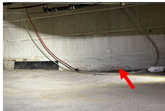
Concrete lintel cracks due to internal corrosion
