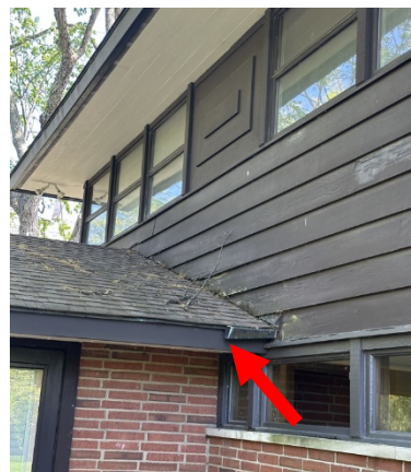
Exterior framing and downspout at west
