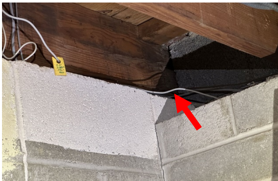
Rim board water infiltration
