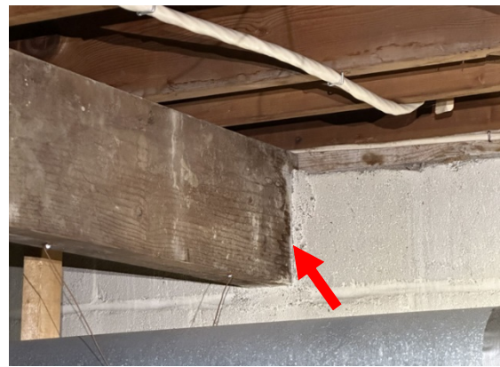
Beam water infiltration at end
