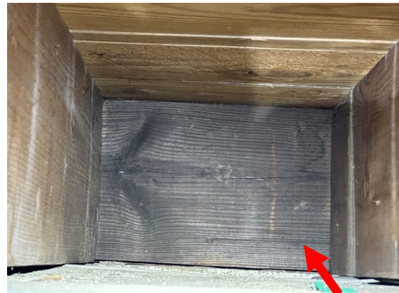
Rim board discoloration
