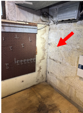
Water infiltration at CMU wall corner
