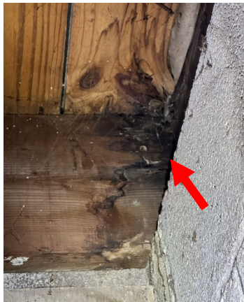
Rim board water infiltration at corner
