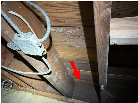
Rim board water infiltration at corner
