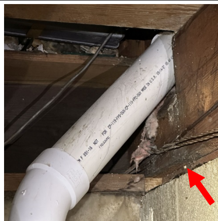
Rim board water infiltration at corner
