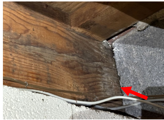
Rim board water infiltration at corner
